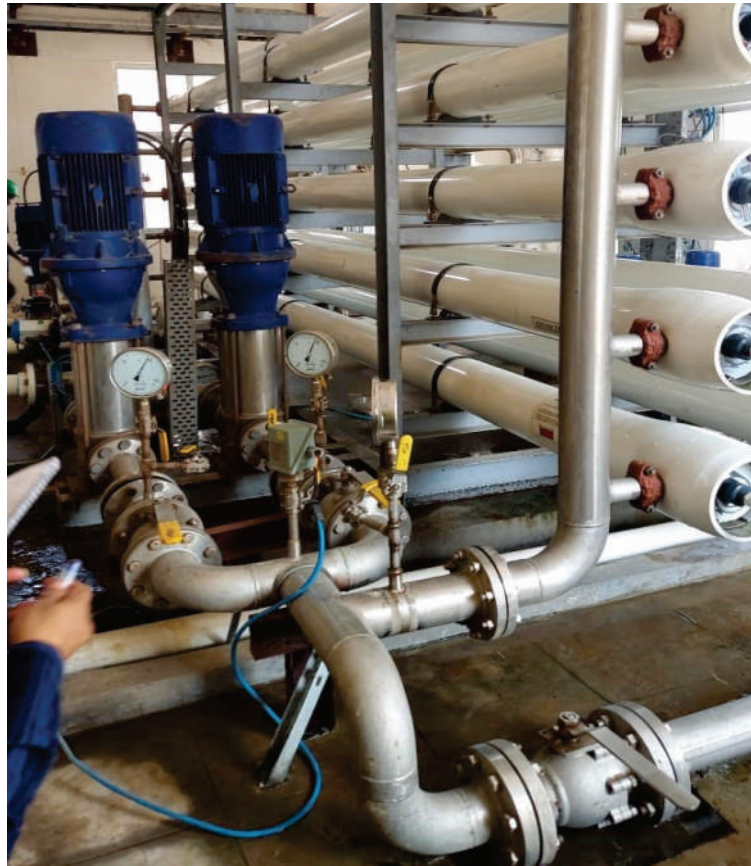
RO based Condensate Polishing Unit
