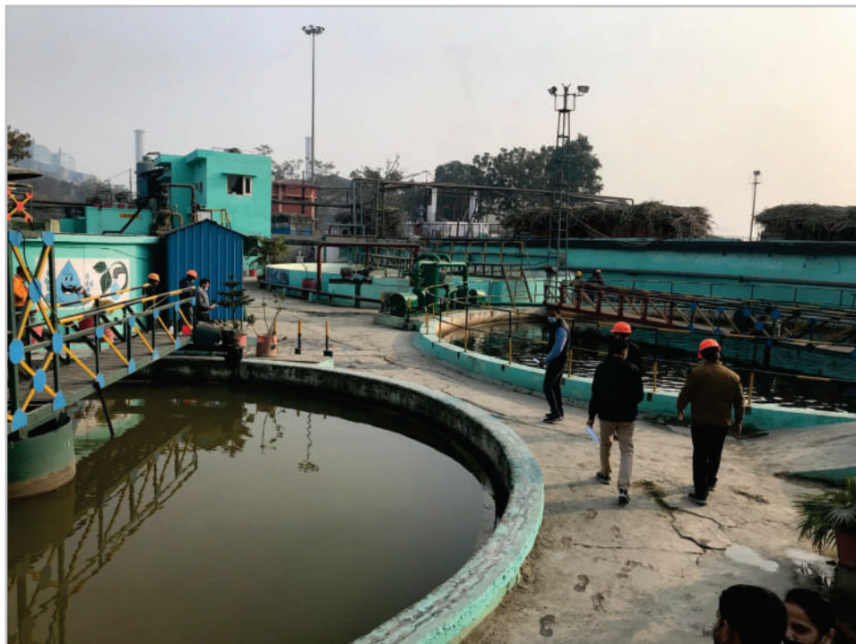
Effluent Treatment plant
